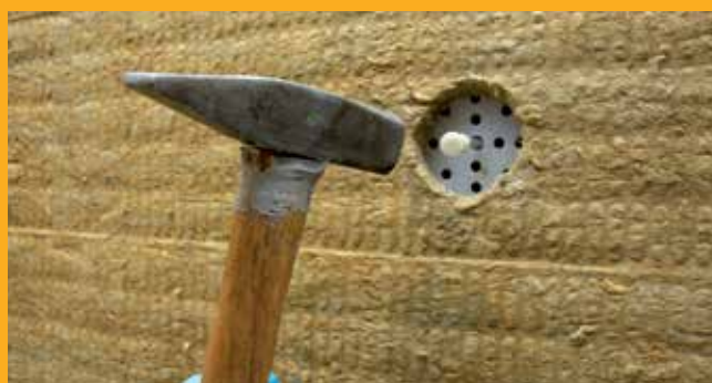
Dodatno pričvršćivanje MW izolacione obloge Additional fixing of MW insulation boards - anchoring
