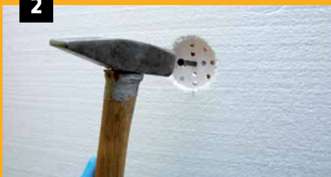
Dodatno pričvršćivanje EPS izolacione obloge Additional fixing of EPS insulation boards - anchoring
